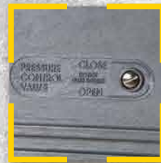
PRESSURE RELEASE VALVE
